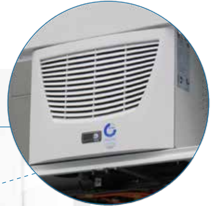
*COOLING UNIT AC TO COOL THE ELECTRICAL CABINET
