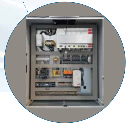
EASY ACCESS TO THE ELECTRICAL CABINET
